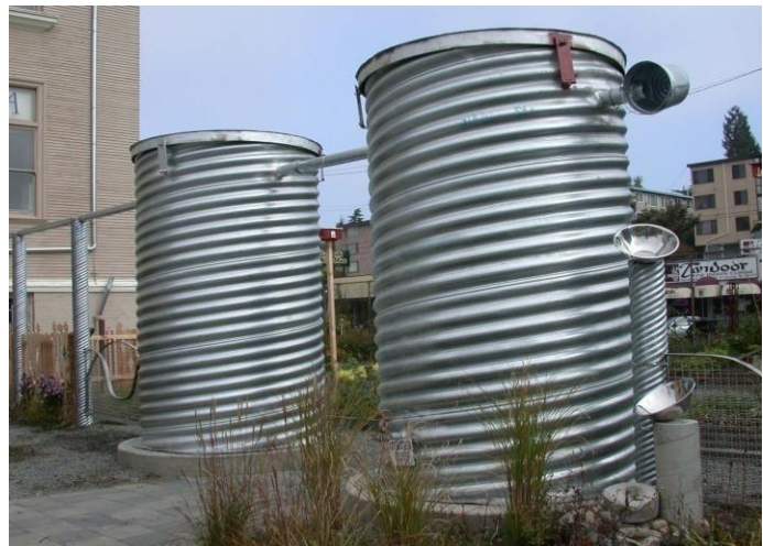
The overflow pipe of this Seattle cistern creates a mini waterfall.
